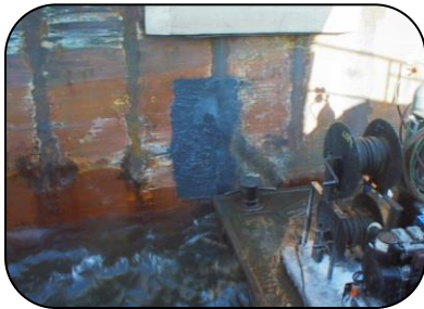
Holed ship hull repaired in sub-zero temperatures using 106 Metal Repair Paste XF and a formed steel plate
